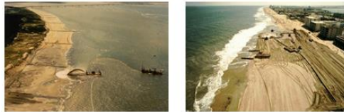
Figure 3.80: Coastal protection through sand replenishment (artificial beach nourishment)
