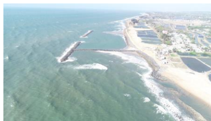
Figure 3.74: Actual construction of the T-shaped groin and 02 breakwater segments to the North
